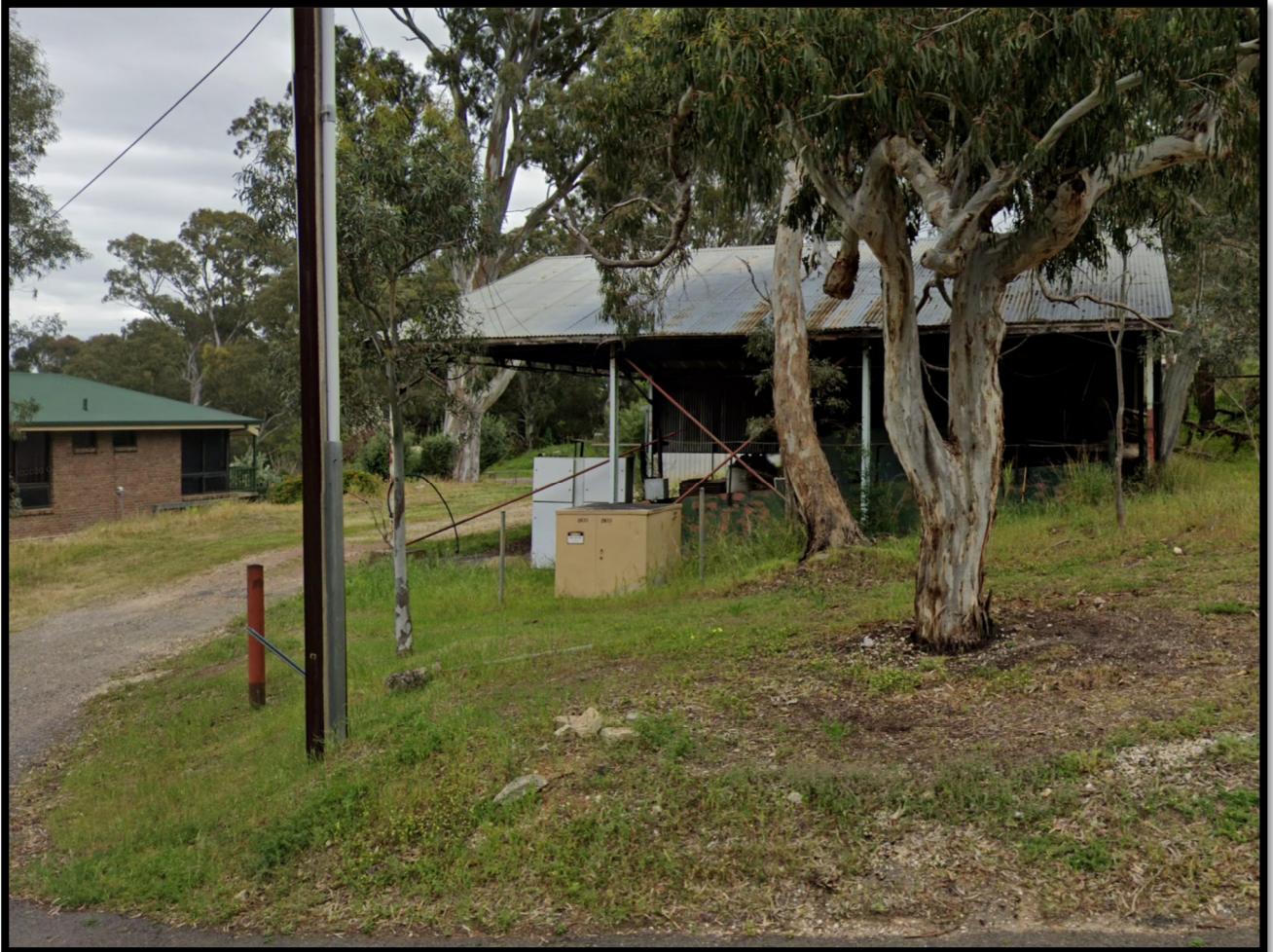
Figure 6 - Transformer adjacent the Halls Road
